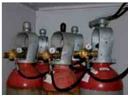
Hydrogen Storage Bay holds up to 5 standard cylinders; enough for >24Hrs of runtime. As an option 8 cylinders can be stored within the room.
